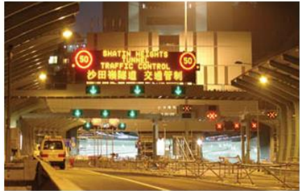
Traffic Control and Surveillance System
